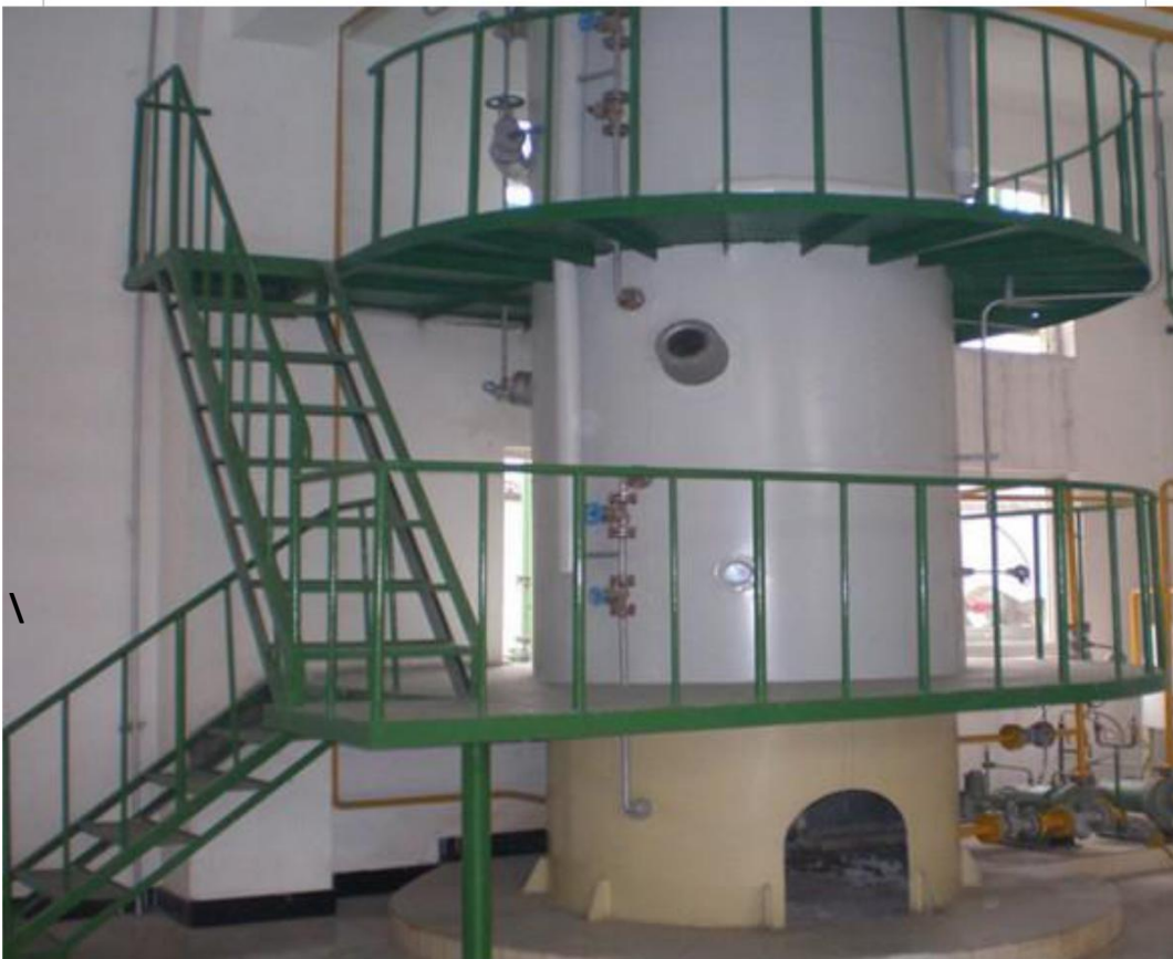
Part of Deodorization Tower
