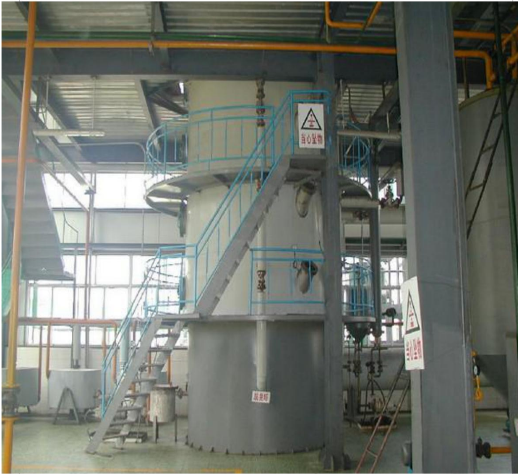
Part of Deodorization Tower
